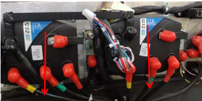
The pump controller
